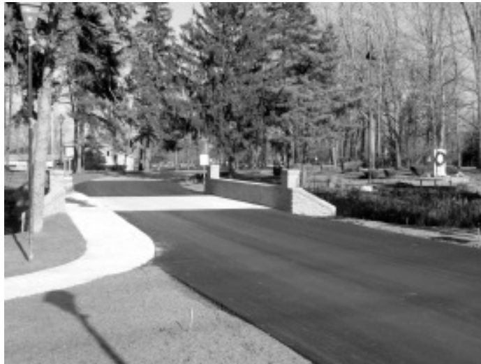
The newly-constructed bridge at the Richmond Heights Community Park will provide a safer route for residents using our parks, school busses and vehicles heading to the Kiwanis Lodge.
